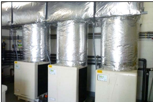
Spa and Pool Heat Pumps
