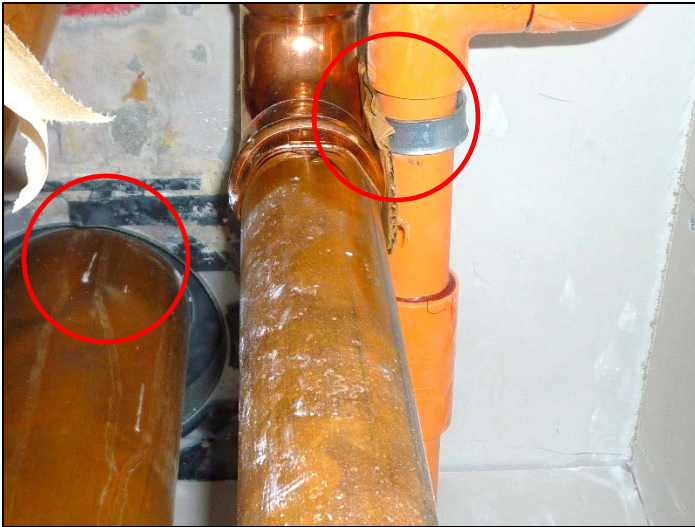
Example of proximity of pipes to one another and to concrete floor.
