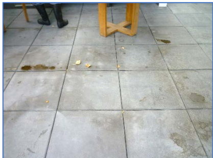
Weekly Scrubbing Before
