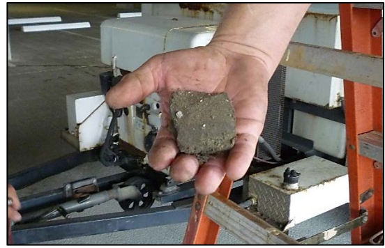
Potential clogging debris dislodged
