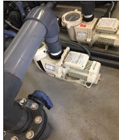
Pool Pump not Lifted off Wet Floor Work In progress
