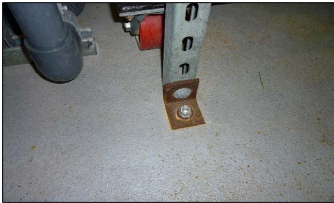
Use of Mixed Metals for Pool Equipment Work In progress
