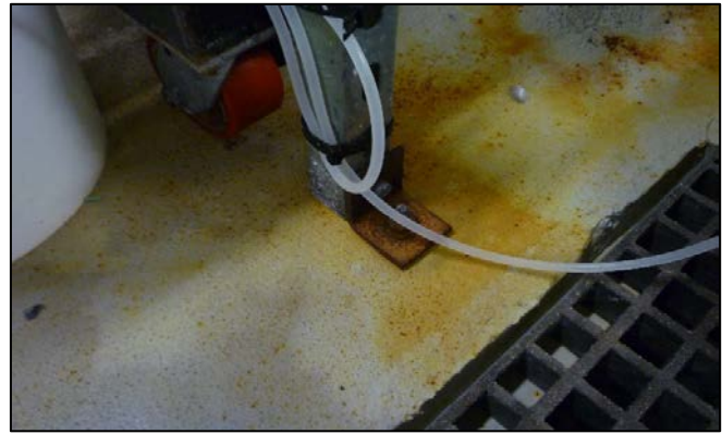
Metal shavings in paint that is rusting Work in Progress
