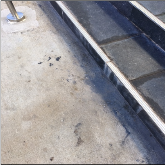
Left Over Grout on Keawe St. Lobby Steps Work in progress
