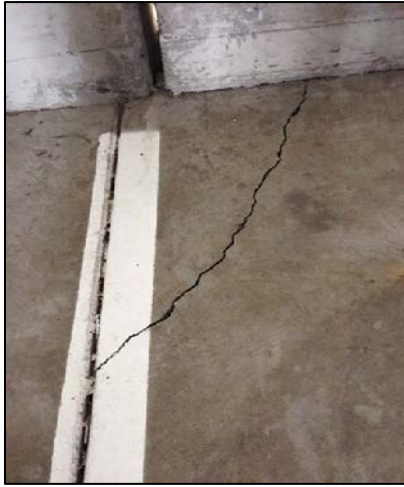
Cracked Parking Stall Completed
