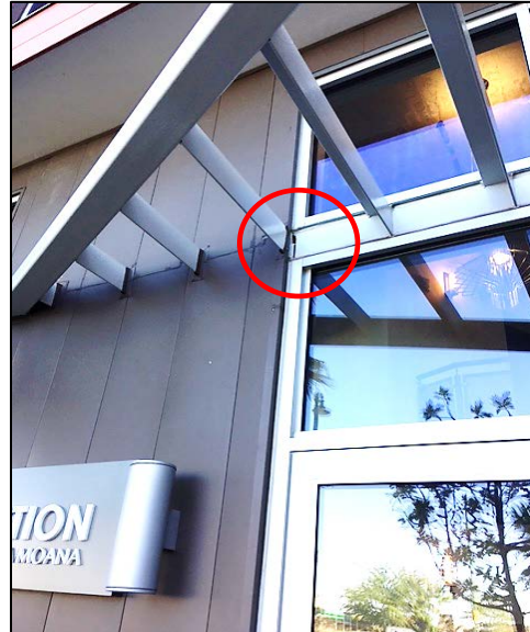
Gap in Lofts Awning - Water Intrusion Possible. Work in Progress
