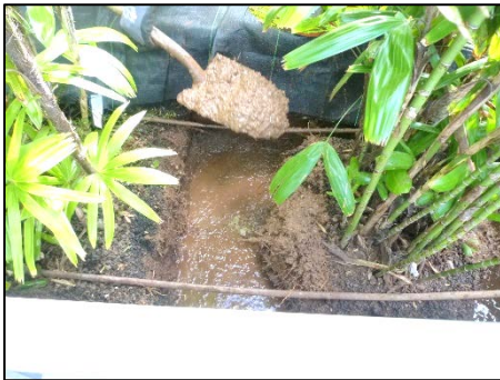
Water Not Draining
