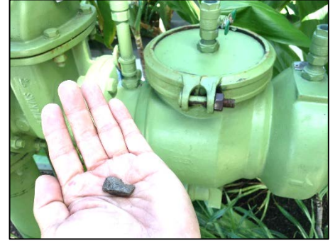
Leak caused by pebble in line
