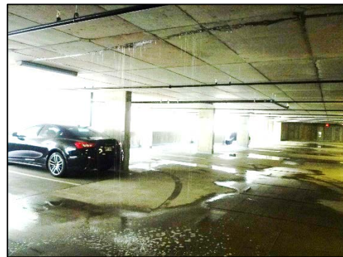
4 th fl Ceiling Leak
