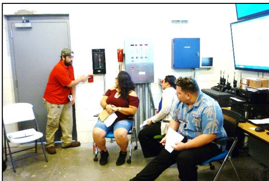
Pull Station Reset
