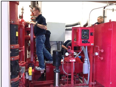
Fire Pump Room Next to Loading Dock
