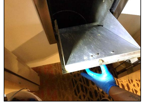
Trash Chute Check (needs to shut after opening)
