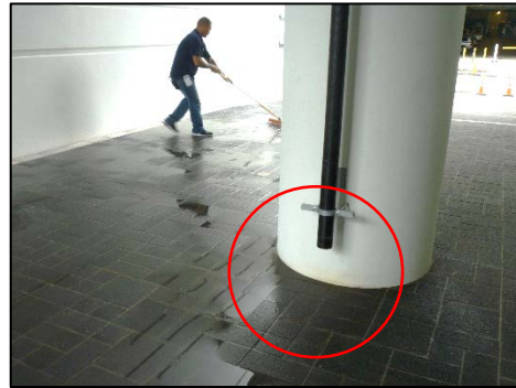
2 Storm Drains terminating onto Porte Cochere
