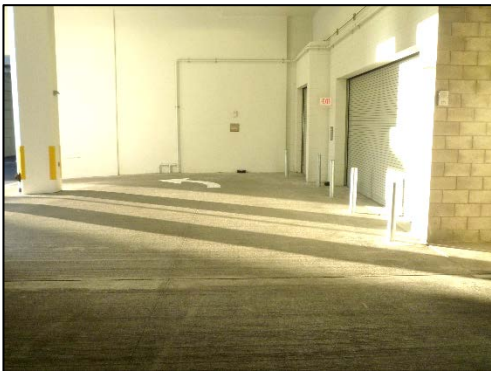
No walkway for Pedestrians
