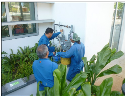
Hawaii Gas Upsizing Gas Manifold
