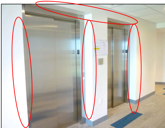
Bare corners at all Lofts Elevator Landings
