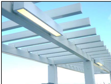
7 th Fl Garage Lights
