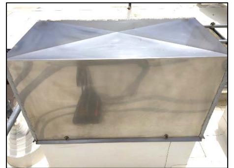
Tower Unit AC Penetration Box After
