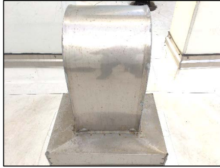
Tower Exhaust Hood Before
