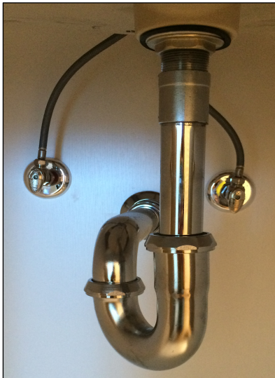
Under-sink water valves
