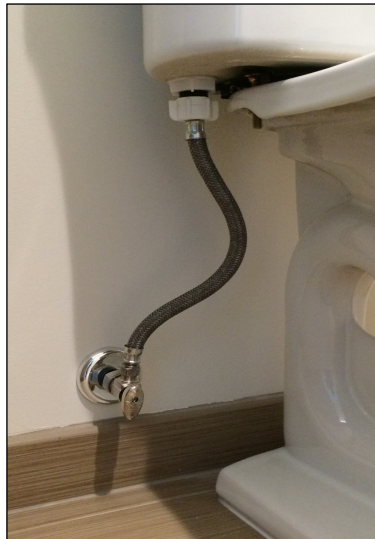
Toilet water valve
