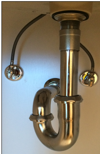
Under-sink water valves
