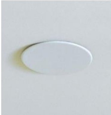
Concealed fire sprinkler in ceiling
