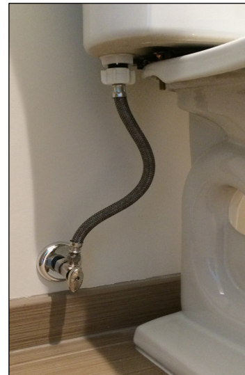
Toilet water valve
