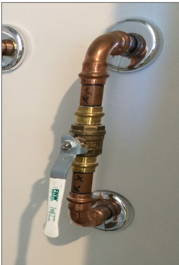
Main water-off valve
